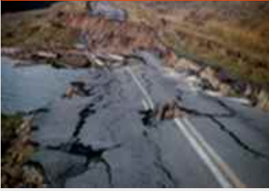
Road damaged due to high rainfall in NE region
